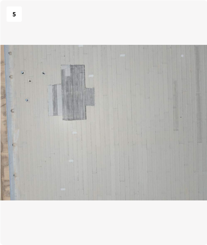
Note patch area Area 2
